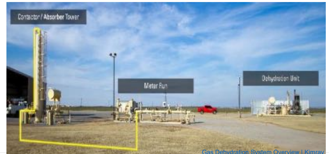
Gas Dehydration System Overview | Kimray
