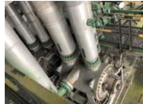
Overview of Gas Compression Facility - EPCM
